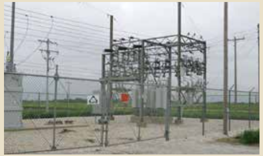
The cathodic protection system protects the copper grounding in the substation as well as galvanized transmission and distribution poles in corrosive soil nearby.
