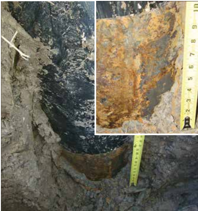
This corroding galvanized steel pole exhibits red corrosion products due to corrosivity of soil, chloride ions and galvanic action.
